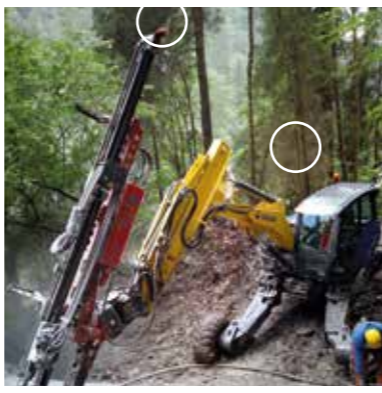
Example of the use of RS193rM* as a fixed point on different surfaces and for the exact alignment of the drill carriage.
