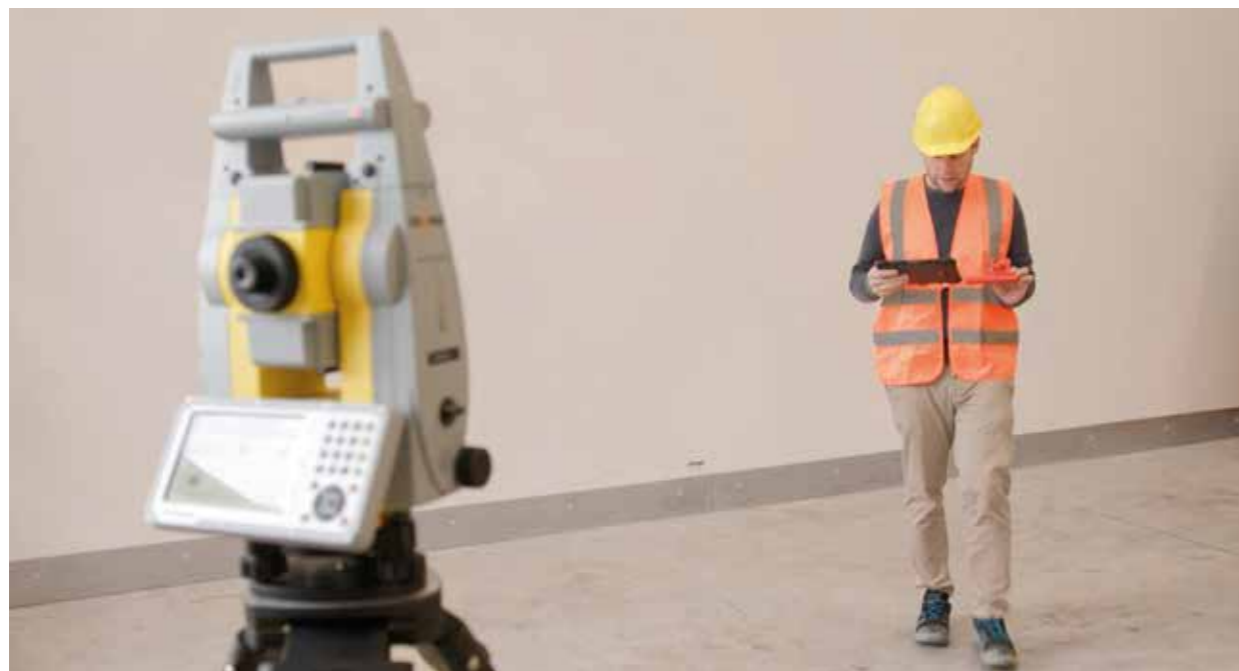
Staking out with the Stake Out Aid for Robotic Total Stations RS150M*
